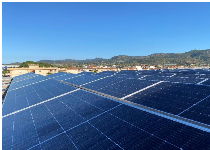
Picture of the solar panels installed at the SanLucar headquarters in Valencia, Spain
